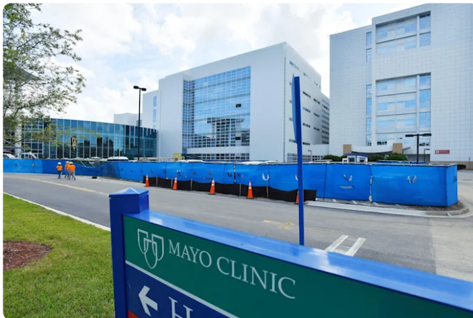
The new wing under construction (center) and the glass-enclosed walkways that connect to the new parking garage are among multiple expansion projects underway at Mayo Clinic Jacksonville.
